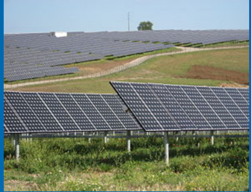
11 MW solar power plant near Serpa, Portugal.
