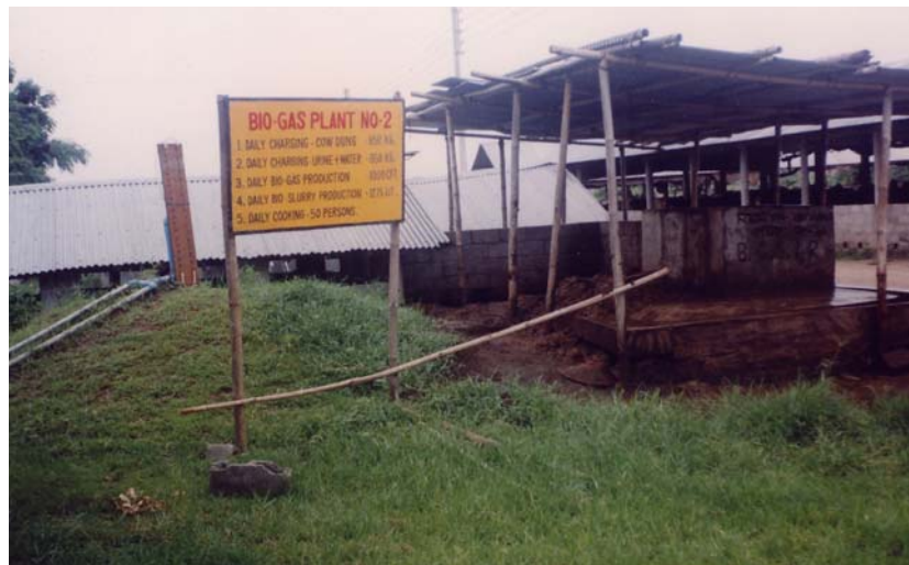
Photo 4.1: Biogas plant with gas delivery pipe at Kazi Tea Estate, Tetulia
