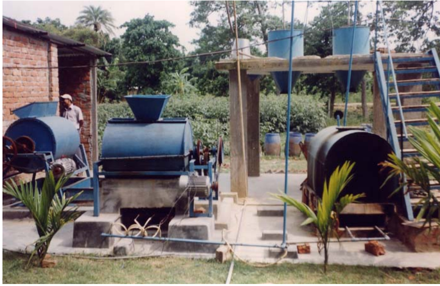
Photo 4.3: Boiler for preparation of poultry feed run by biogas at Raj Poultry Farm, Faridpur
