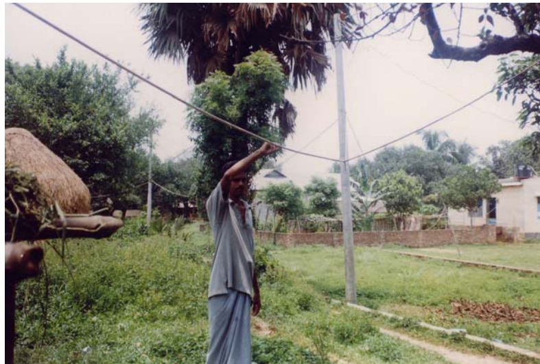
Photo 4.4: Overhead pipe carrying biogas to a neighboring household at Savar
