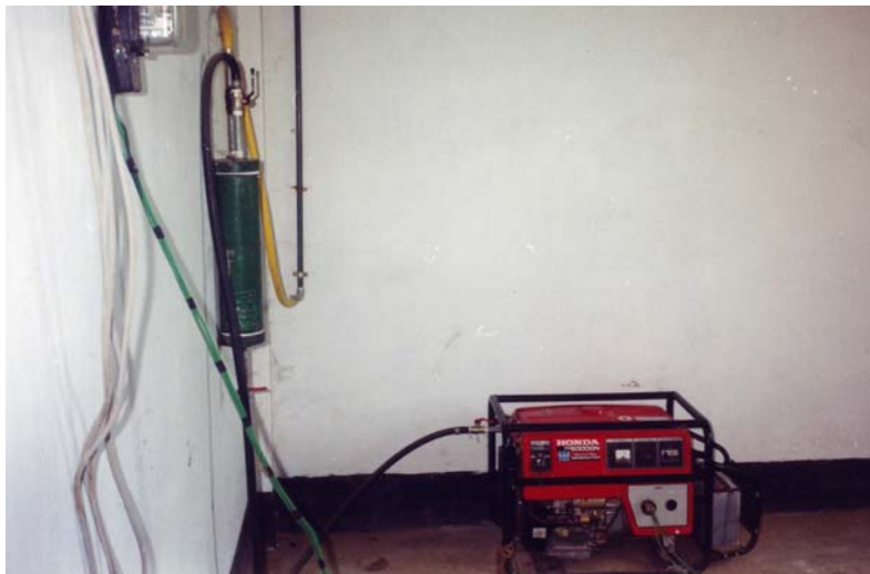
Photo 6.1: Biogas power generator with water trap (hanging on the wall)
