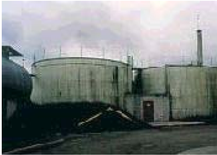
Photo 2.1: Biogas Plant at Wolperthausen, Germany (Gas production: 1800 m 3 /d, Electricity: 550,000 kWh/year)
