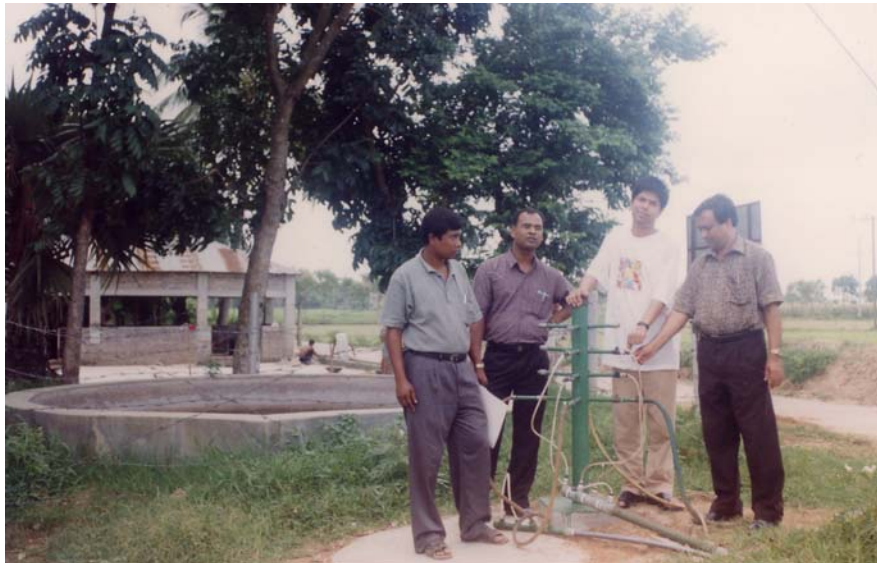
Photo 4.2: Biogas plant with gas distribution lines at RDA, Bogra
