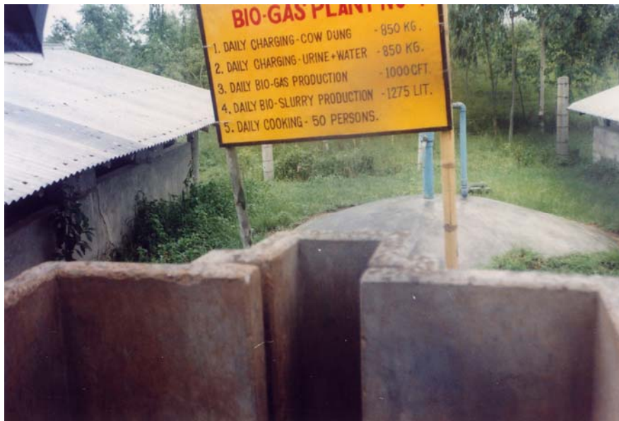
Photo 3.2 : Biogas plant inlet
