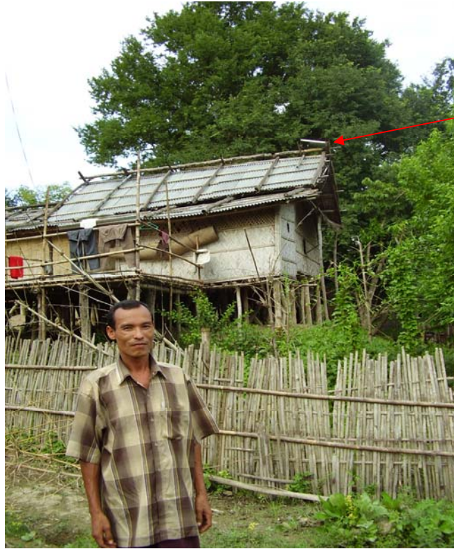
THE SOLAR PV PANEL ON ROOF
