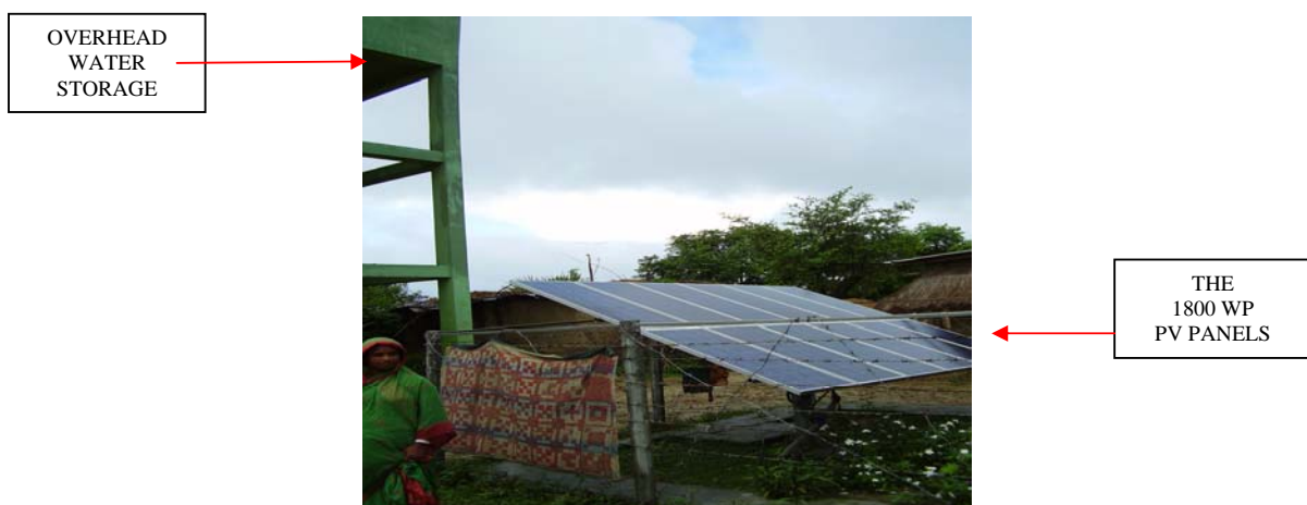
THE 1800 Wp PHOTOVOLTAIC PUMP INSTALLATION AT NACHOLE
