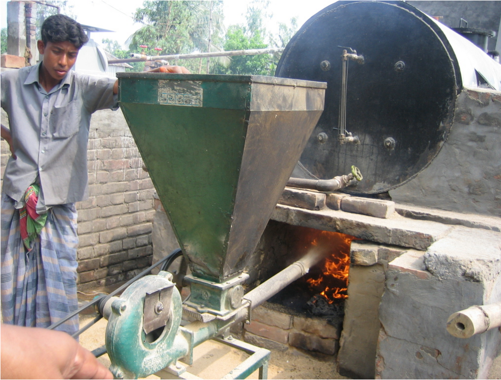
Fig. 12 A view of the steam generation process in running condition at Sherpur, Bogra
