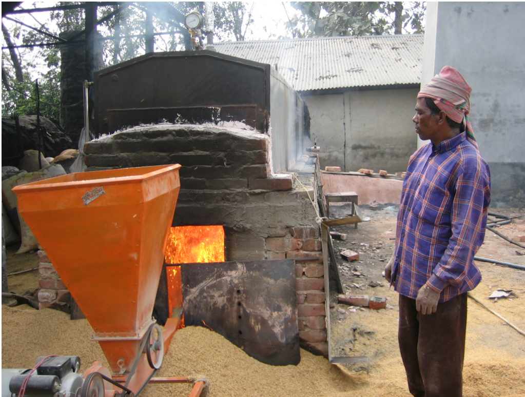
Fig. 11 A view of the steam generation process in running condition showing very good color of flame in the furnace at Kaliakoir, Gazipur
