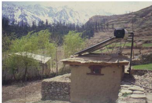
Fig. 10 Solar water heater in rural village in Nepal
