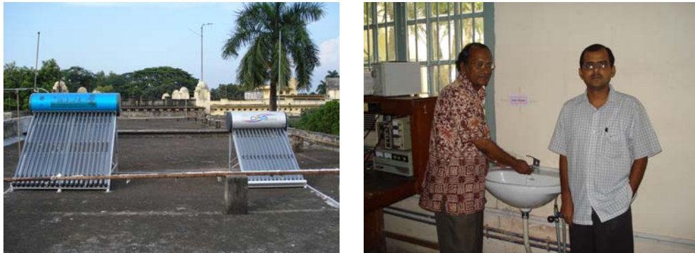
Fig. 5 Solar water heaters at the roof of Old Academic Building
