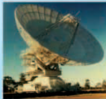
Satellite earth station
