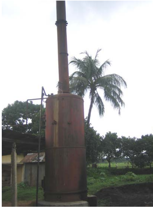
Photo 8. Vertical tubular boiler collected from ship
