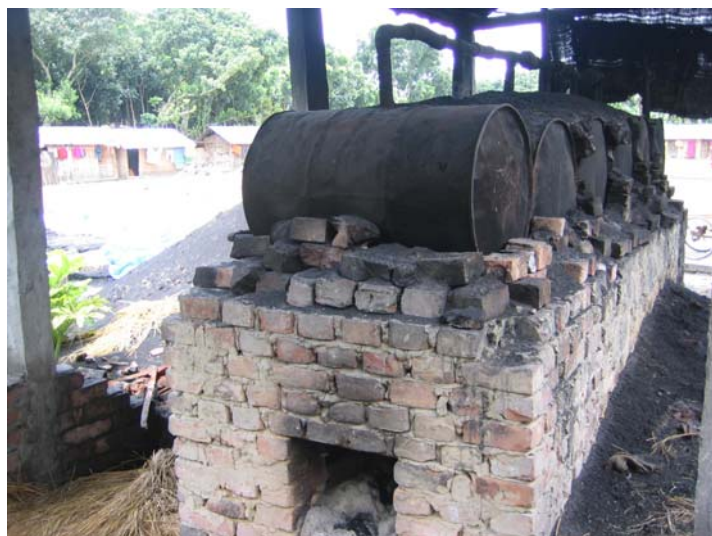
Photo 5. Local made oil drum steam generator
