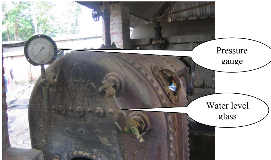
Photo 10. Showing water level gauge and pressure gauge of locomotive boiler
