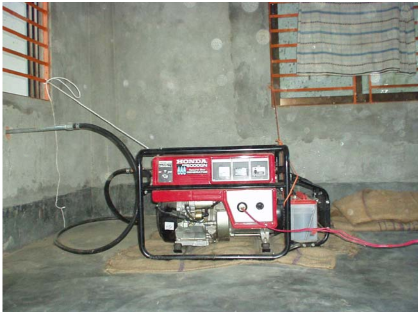
Generator is powered by poultry Biogas at Muslim Mission, Faridpur power generation unit at, Muslim Mission, Faridpur
