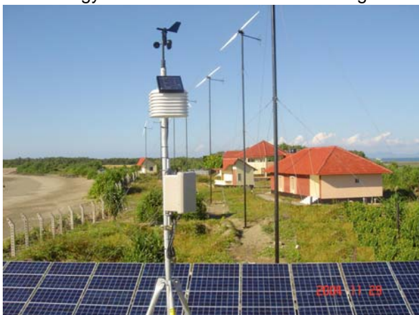
10 kW Wind –Solar Hybrid System at St. Martins Island
